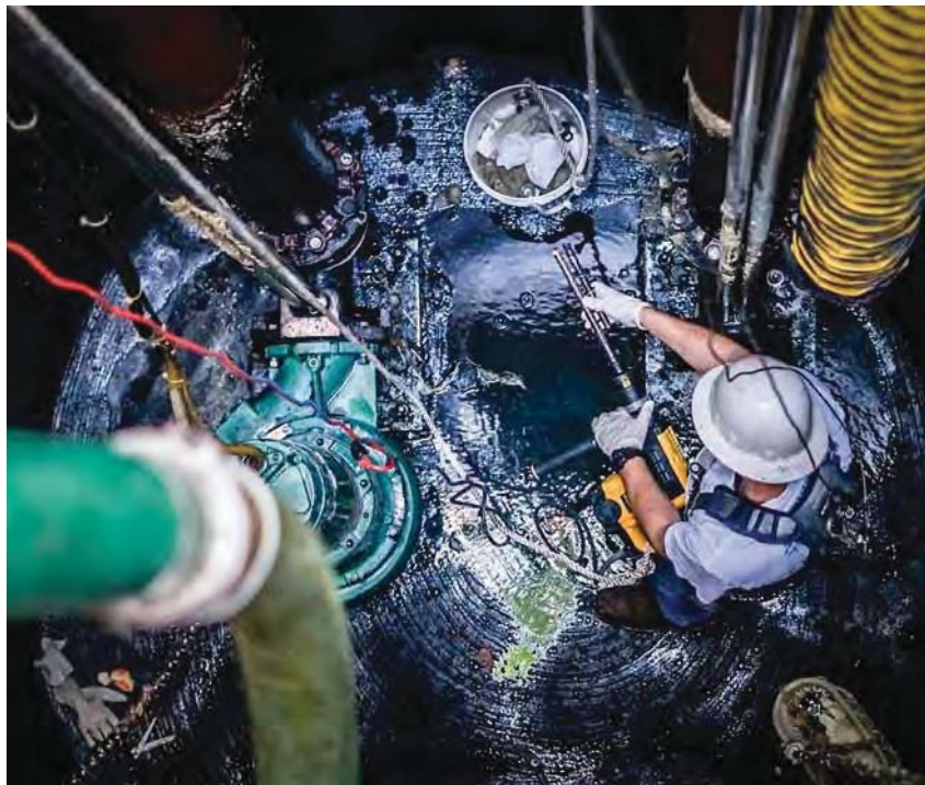
Mike Wisniewski, Utility Plant Mechanic in Lift Station
