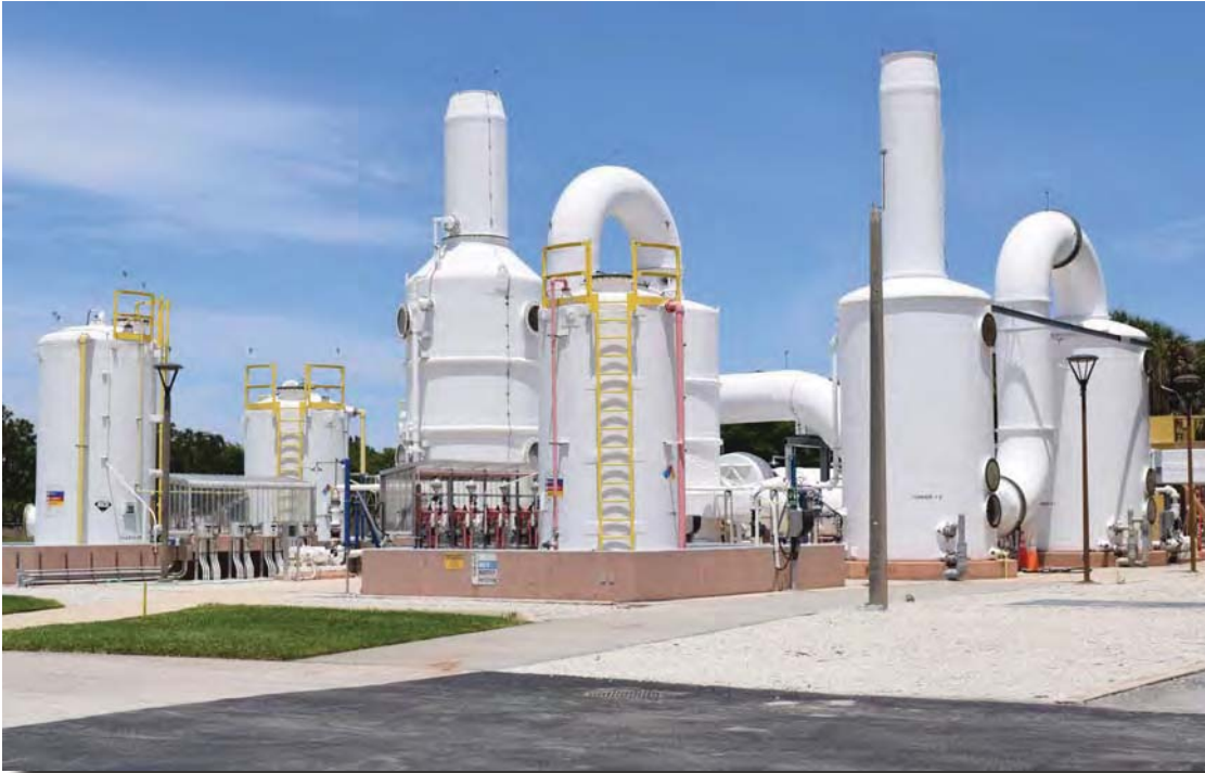
Southern Region Water Reclamation Facility, Boynton Beach
