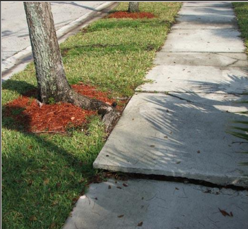
Broken and lifted sidewalks
